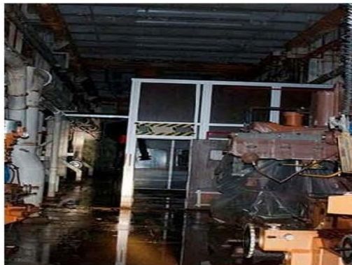
Facility condition and degradation, including standing water and contaminated equipment. (2013)
