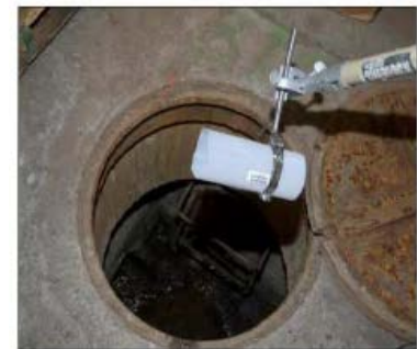
WEMA Storm Sewer Cleanout
