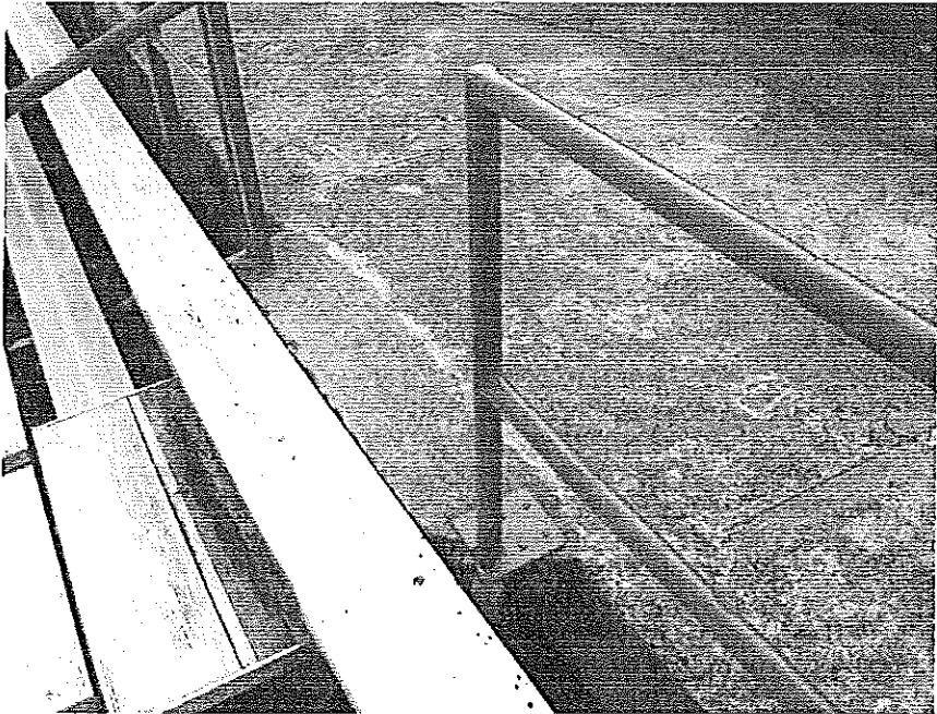
Photo 21: Home Side Metal Bleachers – Cracked/Spalled Concrete at Handrail Connection
