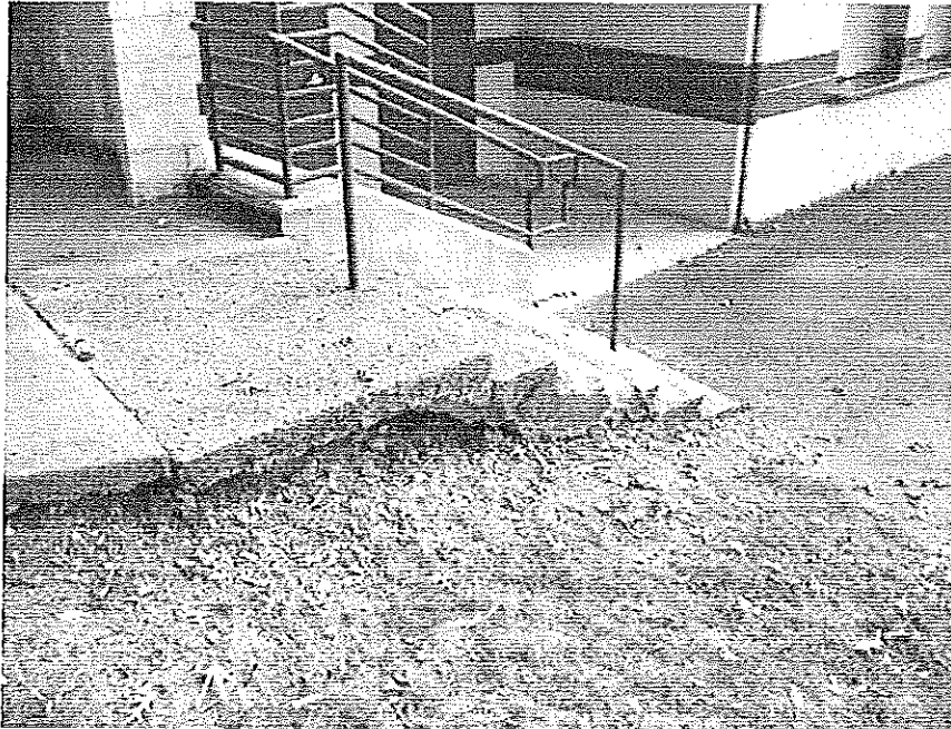
Photo 13: Erosion/Scouring at Stair on Grade – Visitor's Restroom
